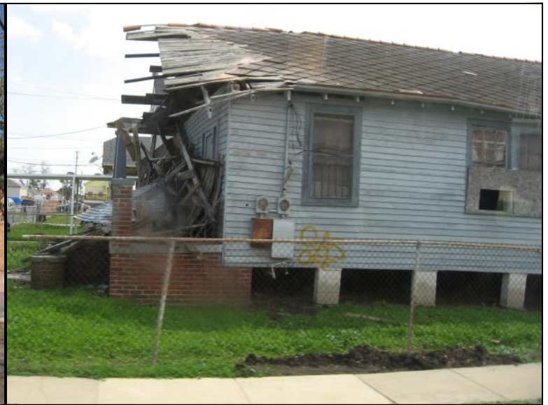
A New Orleans lower Ninth Ward home, ruined by Hurricane Katrina. The community is still struggling to rebuild.
